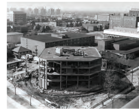
An aerial view of the construction of the building, likely taken in 1974 from the upper floors of the Belcrest Apartments on Cass Avenue. The addition of the Woodcock Wing on the southern side of the structure in 1991 increased the library’s total space by 26,000 square feet.
